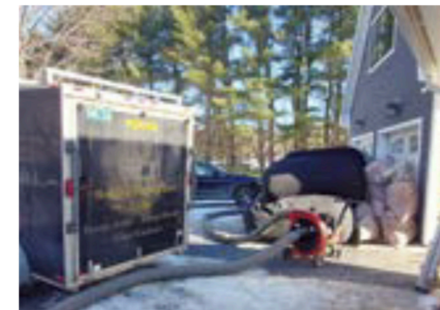
At a typical retrofit project, Sisler's Energy Division vacuums old insulation out of an attic in preparation for air sealing the attic. (Courtesy photo)
